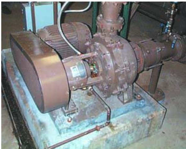
Figure 1: Well Grouted Pump
